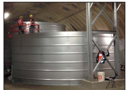
ABB project (Ontario) / made by Aquamerik
