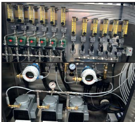
Air distribution control panel
